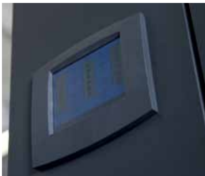
Rack cooling controller display output
